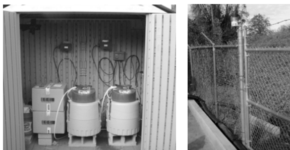
Figure 1. Monitoring equipment shed (left) and rain gage (right) as installed at the monitoring site.
